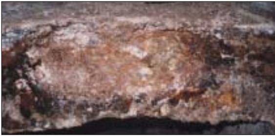
Bottom side view of 12-inch x 12-inch x 6-inch (30-cm x 30-cm x 15-cm) reinforced concrete steel beam in wet well. Six years' service in Louisiana wastewater treatment collection system. Concrete loss is greater than 4 in. (10 cm)
