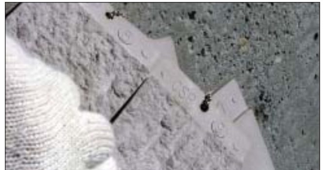
Concrete comparator panels from ICRI being used to determine adequacy of surface preparation
