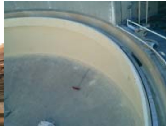
(above) Gravity thickener tank (rehab.) lined with 20 mils (1/2 mm) of epoxy (left) Underground clarifier lined with 1/4-inch (6-mm) epoxy mortar Photos courtesy of the author
